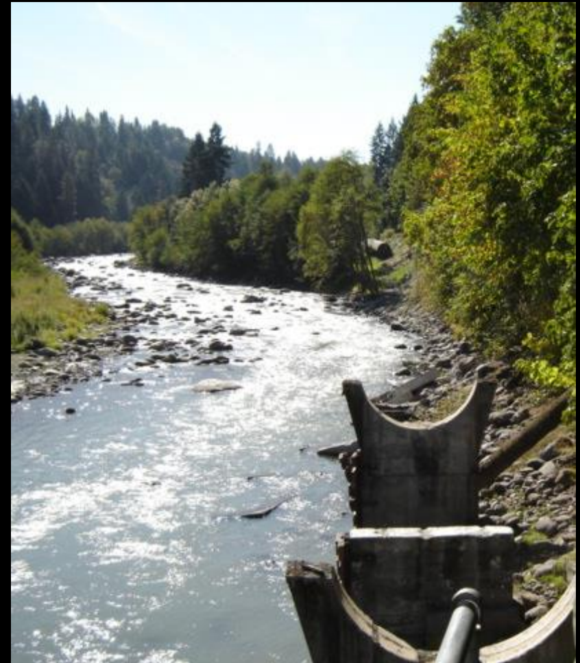
A large section of pipeline delivering water to the powerhouse were destroyed in 2006 debris flow
