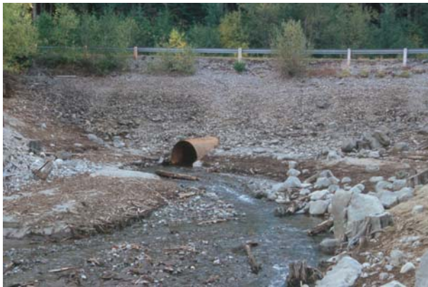
Photo Left: A culvert at the mouth of Pinnacle Creek entering Laurance Lake during low reservoir pool elevation creating a fish passage impediment for bull trout.
